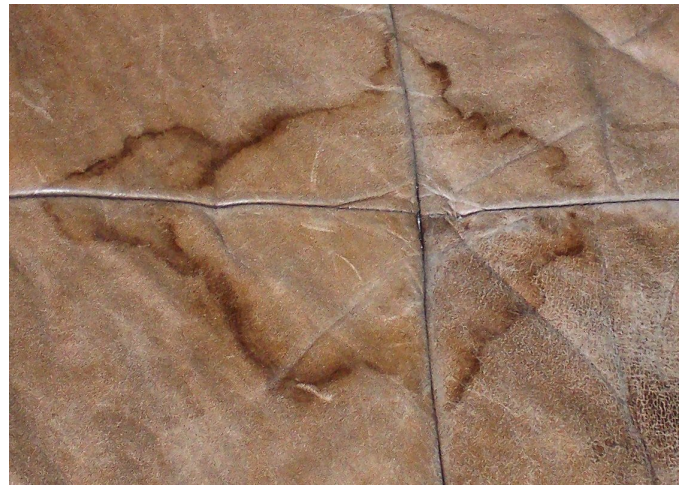
Penetrated stains: Standard cleaning attempts will not work.
